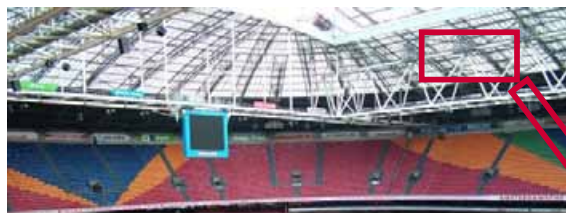
Area where sheets were removed for evaluation
